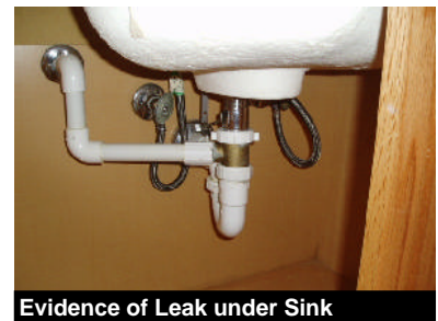
Evidence of Leak under Sink
