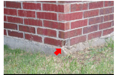
Broken Brick Course at Back Patio
